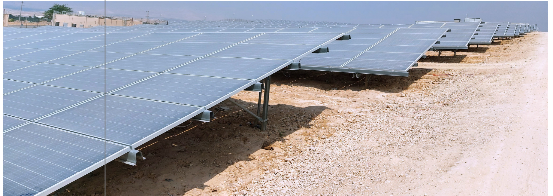
Kabad Photovoltaic Plant
